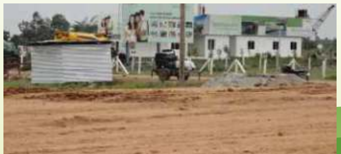
6 lane express high way - Work in full swing in front of Brindavan site
